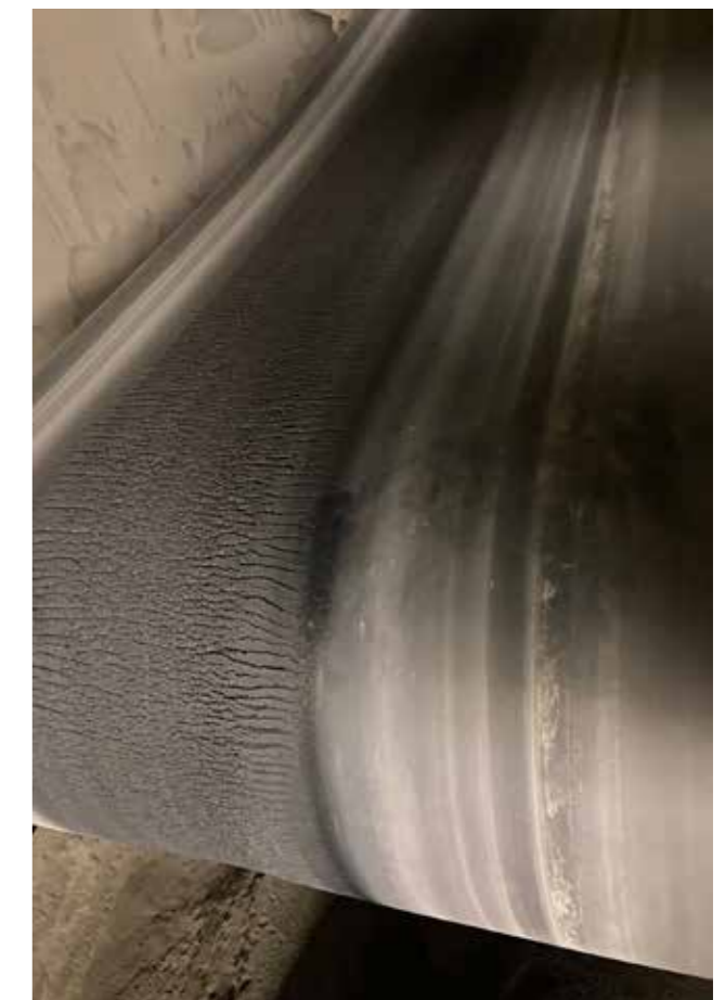
Cracking up. Without ozone and UV resistant covers, wear and tear is accelerated.
