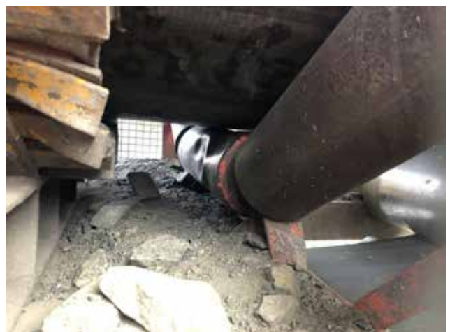
Unclean environments and damaged rollers can accelerate wear.
